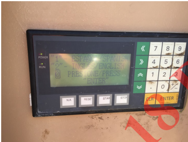
Ojo de Agua Self Service Water Dispensing Facility
